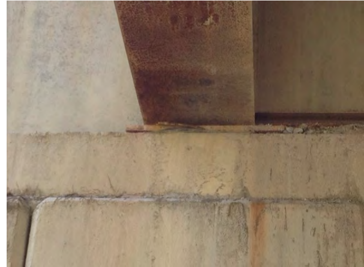
right downstream bearing pad keeper separating
