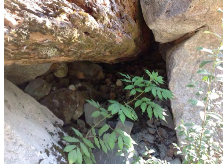
voids in left upstream abutment
