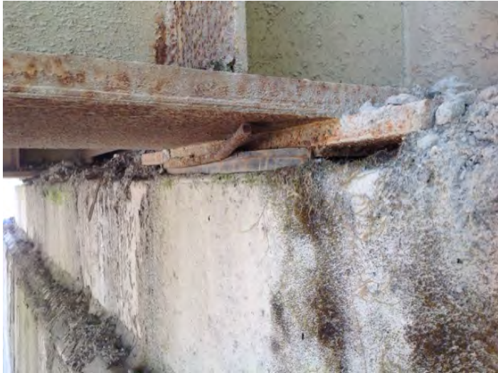
right upstream bearing pad keeper separating
